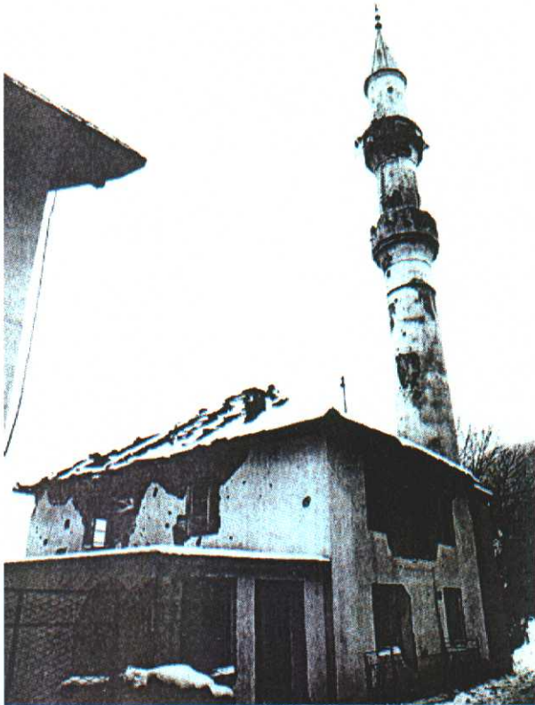
photo from: K.Zukic, Slike zlocina (1999) - note projectile damage to perimeter walls and roof, shell holes in minaret
