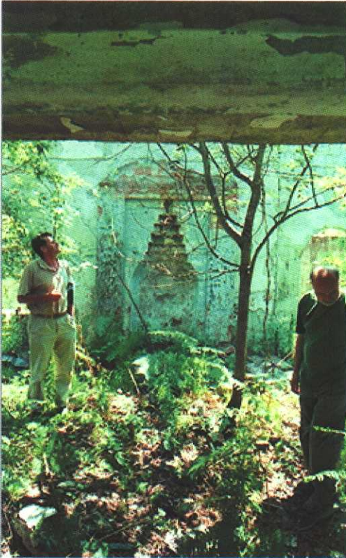
photo by: András Riedlmayer (07/2002) - gutted interior of Drinjaca Mosque, with prayer niche ( mihrab )
