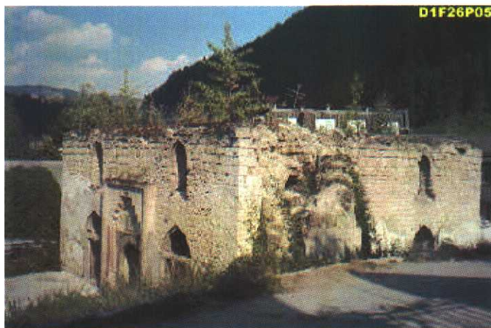
photo from: Council of Europe (1998) - remains of Sinan Beg Mosque as of 1998: minaret blown away, dome and roof gone
